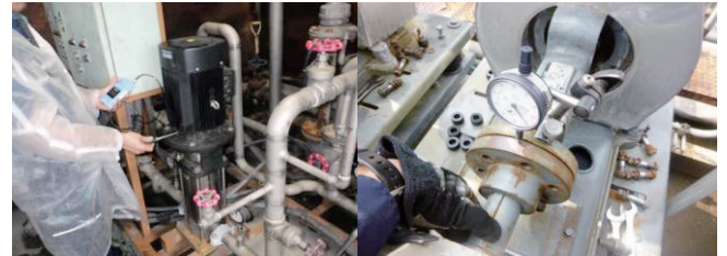
Fig. 2. Photograph of the inspection of the control system of the RIBF water-cooling system.
