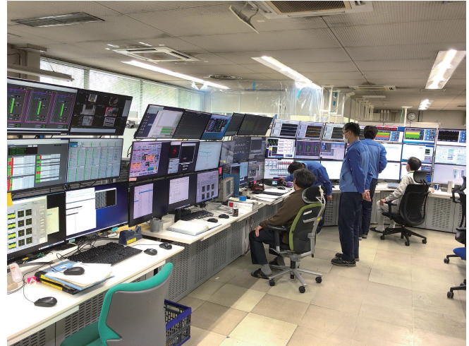
Fig. 15. New consoles for remote operation in the RILAC control room.
