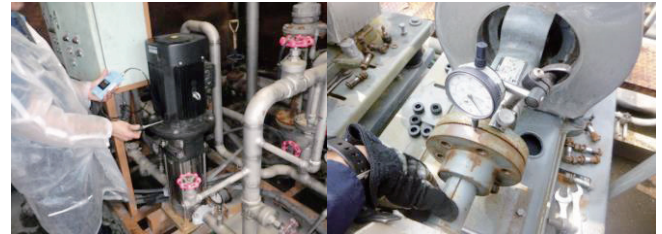
Fig. 2. Photograph of the inspection of the control system of the RIBF water-cooling system.
